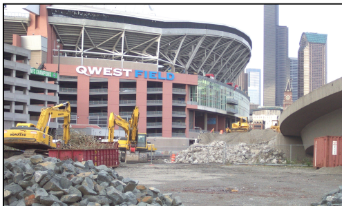
Demolition of the former 4 th Ave. I-90 on ramp in underway in November. The work will make way for relocation of the BNSF mainline south from King Street Station. Photo by Warren Yee
