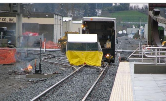
In March, Sound Transit's contractor is working the rail reconstruction project at the future South Tacoma Sounder Station, near South 60 th St. Amtrak service will eventually share this route with Sounder. Photo by Jim Hamre
